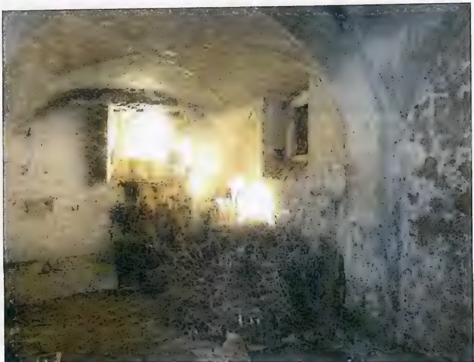
The house is a complete ruin but remarkably it still stands 70 years on.
